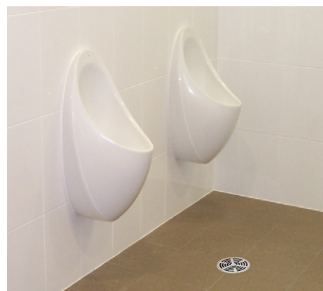
Photo 1: Typical floor waste gully for wall hung urinals
